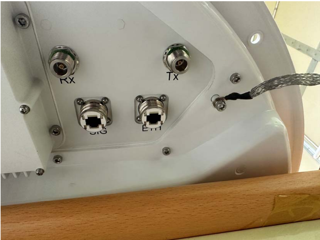
(located at Bottom of Antenna)
