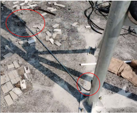
The holding pole lightning rod is not led to the ground bar
