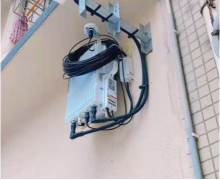
GPS antenna blocked
