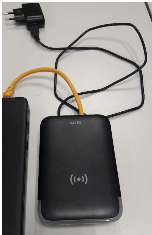
Photo 6: Ethernet connection + Power supply
