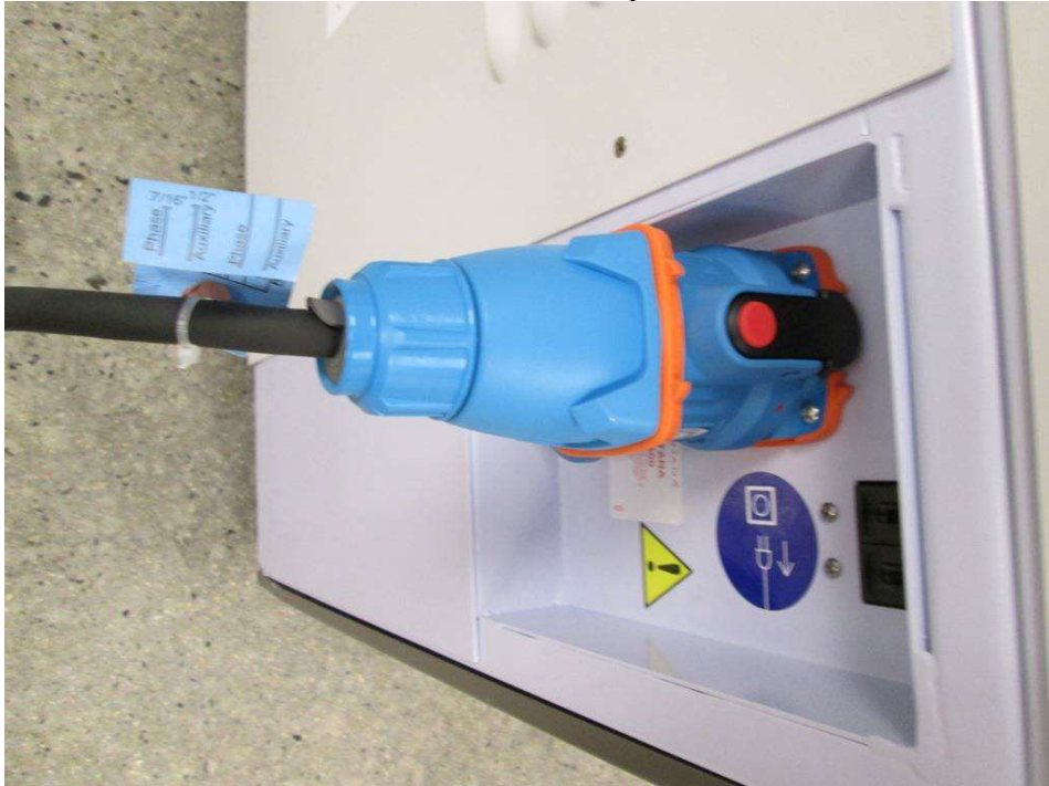
Photo 7: Ventana HE 600 Mains power connection
