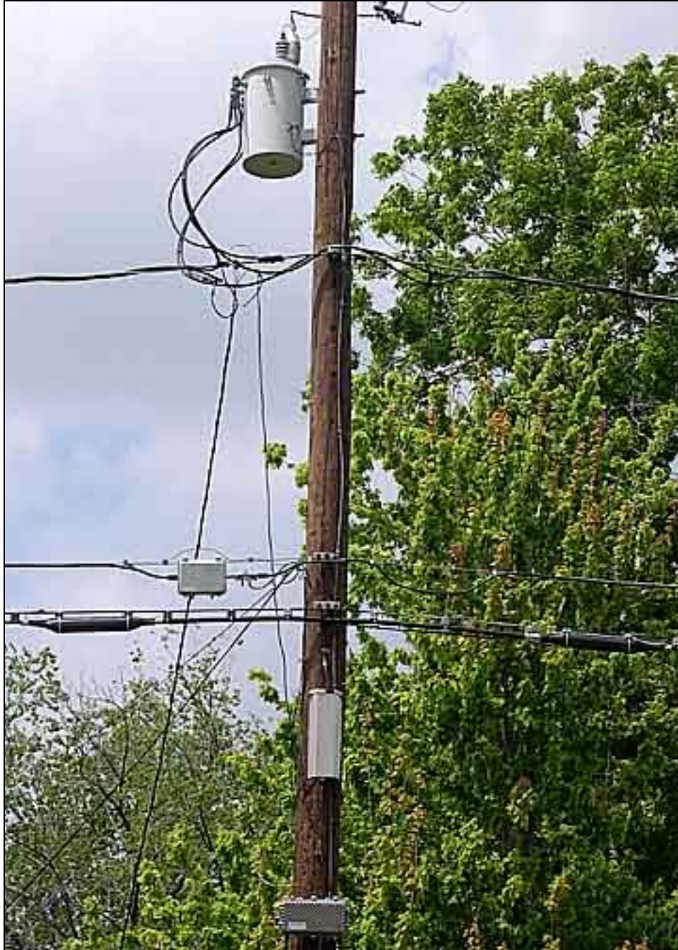
Unit Installed on Pole
