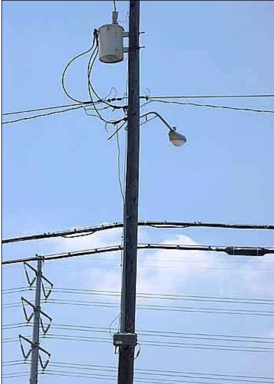
Unit Installed - Closeup
