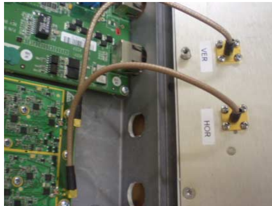
Photograph 7.7.3 Antenna assembly, integrated
