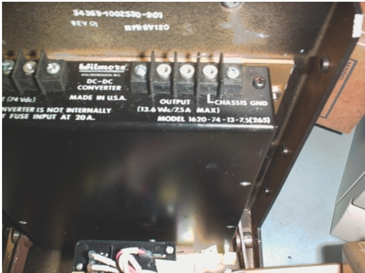
Photo H.13 Wilmore DC-DC Converter
