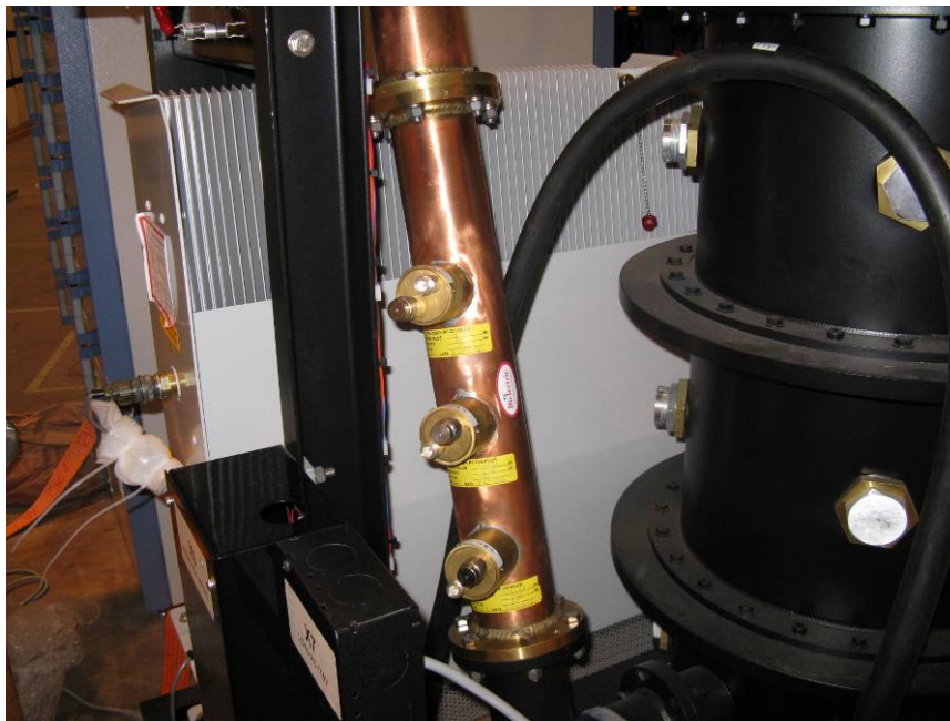
Figure 6-8: Picture of Power Coupler
