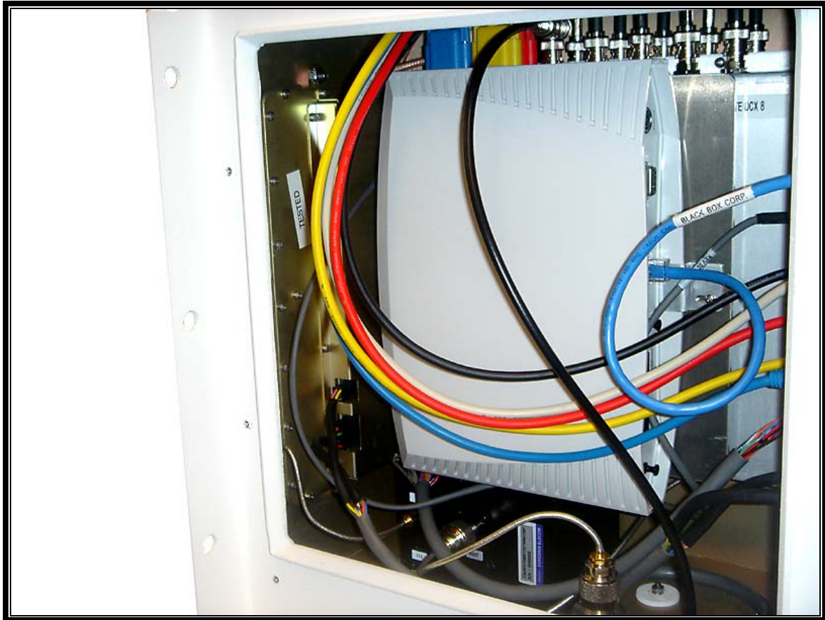
Photograph 10: Cell Site Interior – Back View
