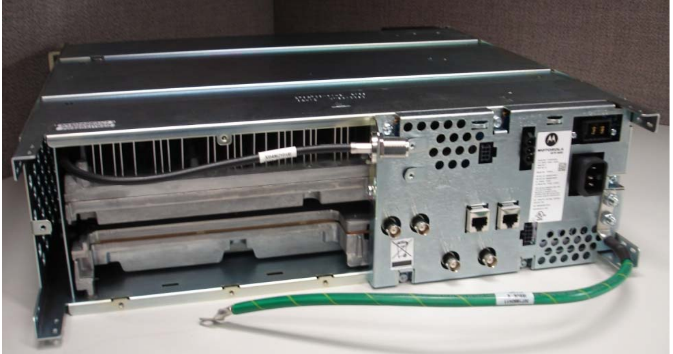
External Back View of Base Radio
