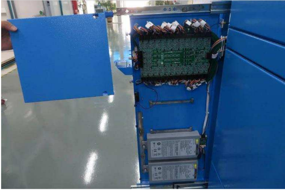
Internal view with 2pcs batteries
