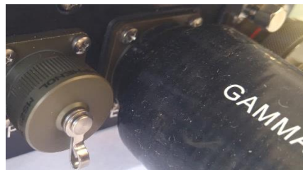
Figure 12: Collapsing Cold Shrink
